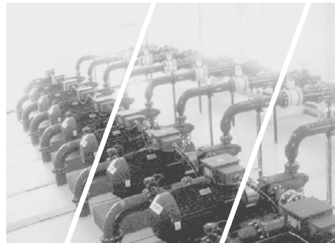
Boosting and Distribution of surface water
