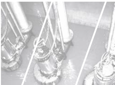
Wastewater Transport and Treatment
