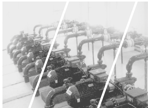
Boosting and Distribution of surface water
